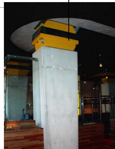
Spring element in dressing-room area
